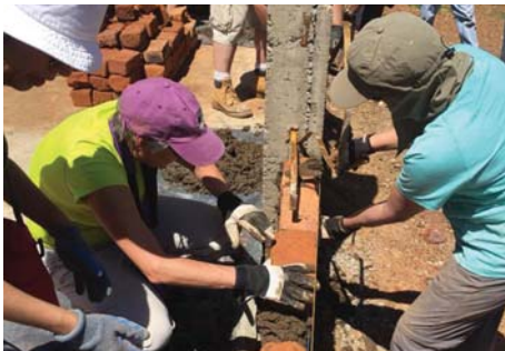
Paula Vogler in yellow and Renita Turner in blue laying bricks on the first day of construction.
